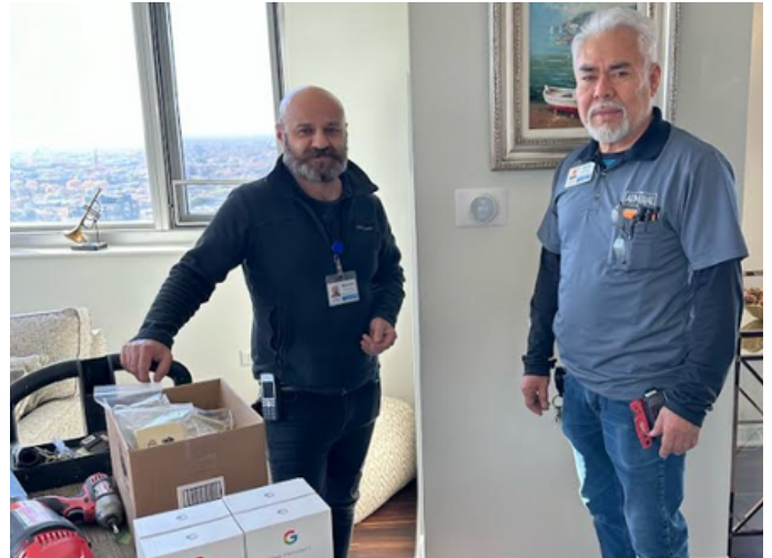
Martin Khoshaba, Lead Maintenance Technician, and colleague Jerry Vazquez install one of the new smart thermostats.
