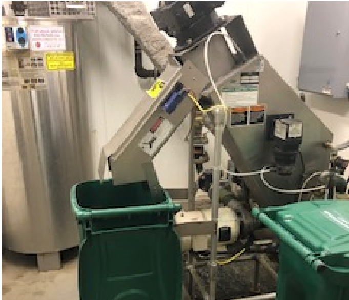
Slurry is fed to the Somat pulper where de-watered and semi-dry pulp is fed into a haul-away container.
